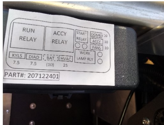
FIG 2A-HVAC FUSE LABEL
